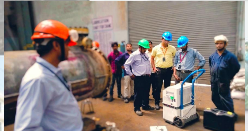
Helium Leak Testing of Heat Exchanger being done
