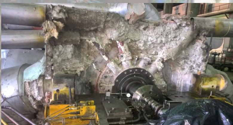
Turbine of 210 MW unit at Kota. Borescopy & UT was done
